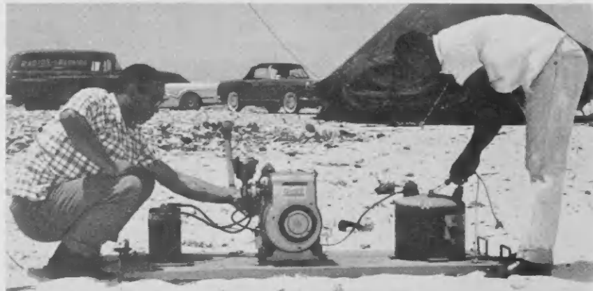
SETTING A portable generator in place at the Palm Beach site was the task of Joe Cijntje and Calvin Colbourne. Station PJ3AL was located at this position under the direction of Max Sand.
